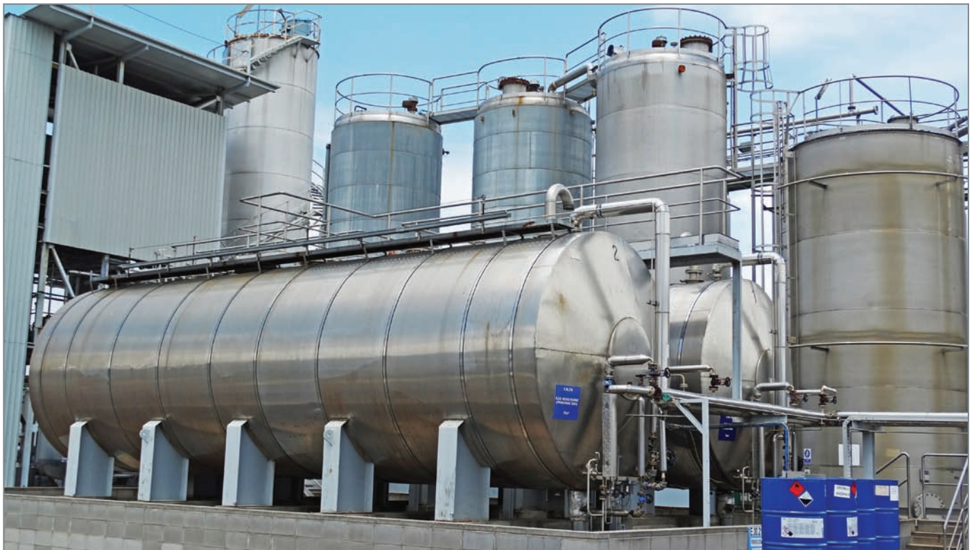
The CRODA Mevisa site celebrated 20 years of operation in 2018 and Almatec® AODD Pumps have played a major role in ensuring the plant's success.
