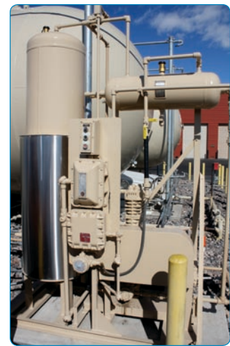
Vapor-recovery unit currently in use at YCS facility, featuring an LB161 Series Compressor from Blackmer.
