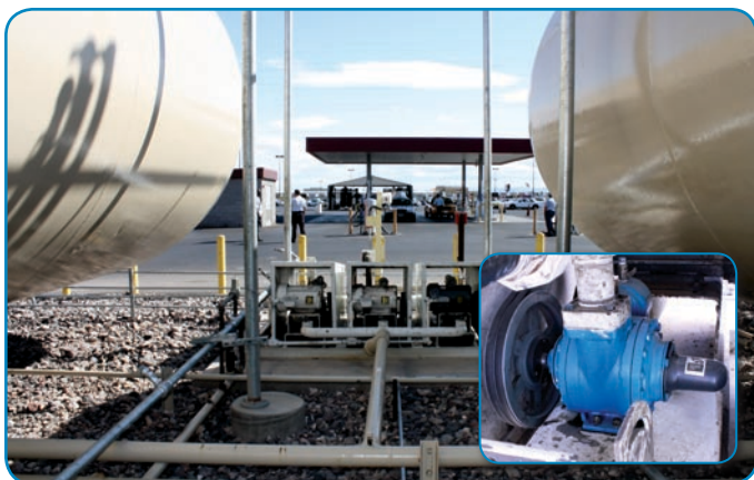
The facility replaced 6 pumps with 3 LGLH2A pumps. Blackmer pumps were chosen due to their reliability, cavitation suppression and ease of maintenance.
