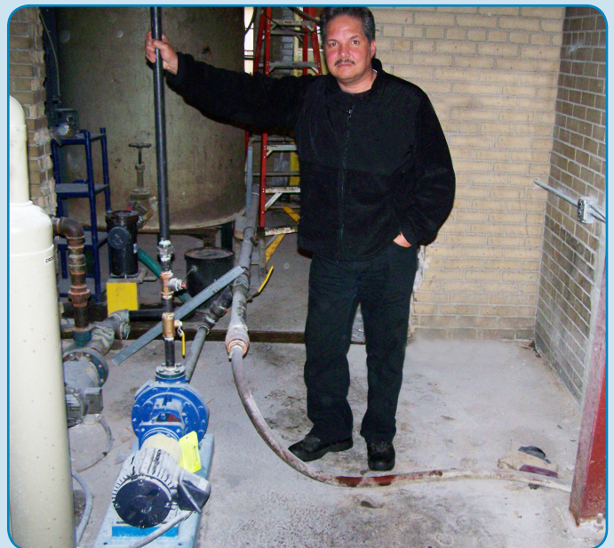
Santos Flores next to the trouble-free Griswold 811 ANSI Series centrifugal pump in a cooling application.
