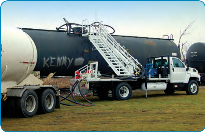
This transloading application features Blackmer compressors transferring LPG from railcars to transports.
