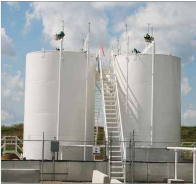
In-the-field storage tanks are used to house raw crude oil and natural gas before it can be transported for refinement. Operators must control the amount of potentially harmful vapors that are released to the atmosphere from the tanks and are turning to vapor-recovery units as a solution.
