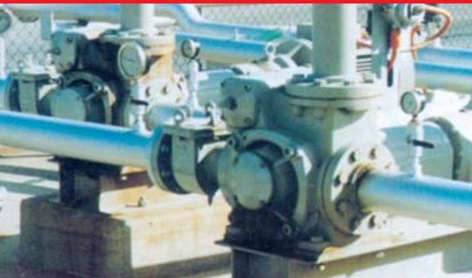
Oil Terminal load in/load out
