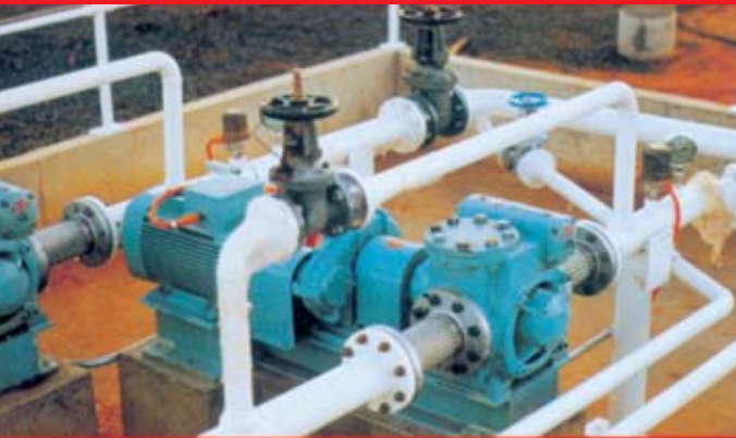
High Capacity rail tank car unloading
