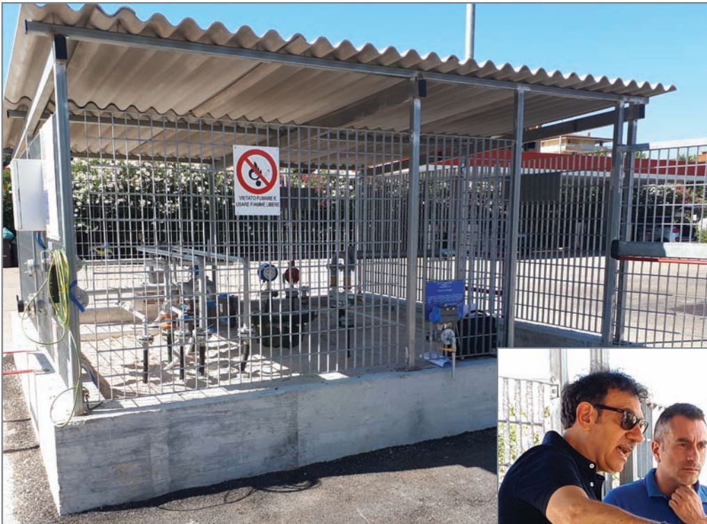
The limited amount of space at the fueling site, left, required the installation of a vertical 25,000-liter UST, which uses an electric motor that can produce 2,900 rpms during the Autogas-dispensing process.
