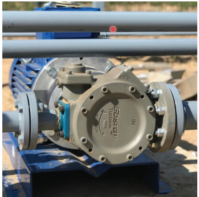
A regenerative turbine pump pumping hydrocarbons in a chemical plant.
