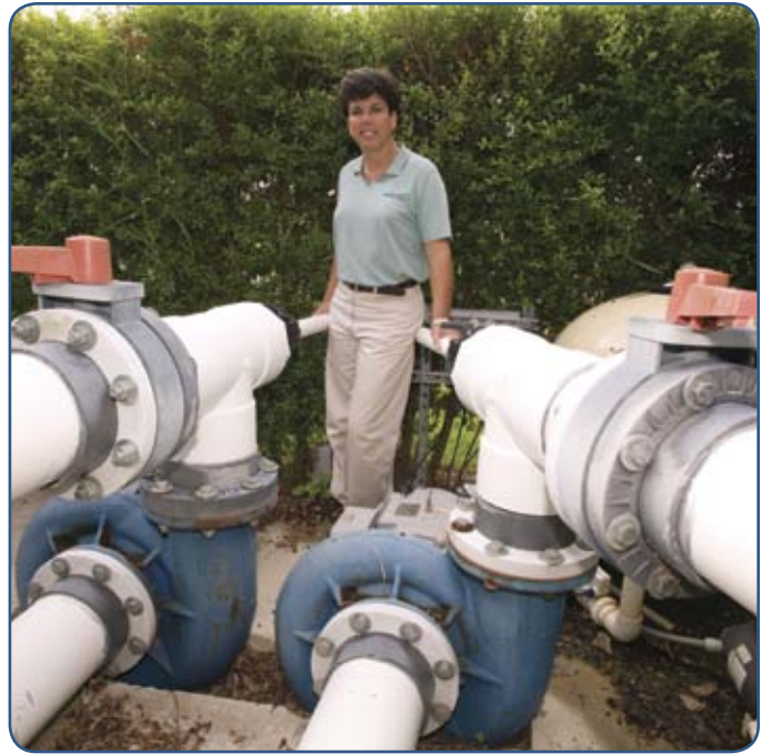
HeartSong WaterScapes relies on Griswold E,F&G Series centrifugal pumps for all of its waterfeatures. The Griswold pumps pictured here have been performing perfectly for 14 years at the Canyon Isles housing development in Boynton Beach, FL.
