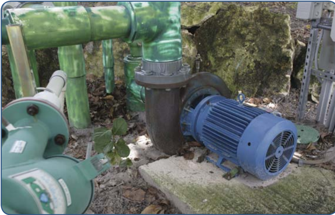
Griswold E,F&G pumps meet the needs of HeartSong WaterScapes because they are designed with enlarged suction and discharge nozzles that cut down on friction losses, making them ideal for water-pumping applications. The Griswold pump pictured is located at the Valencia Isles' waterfeature.
