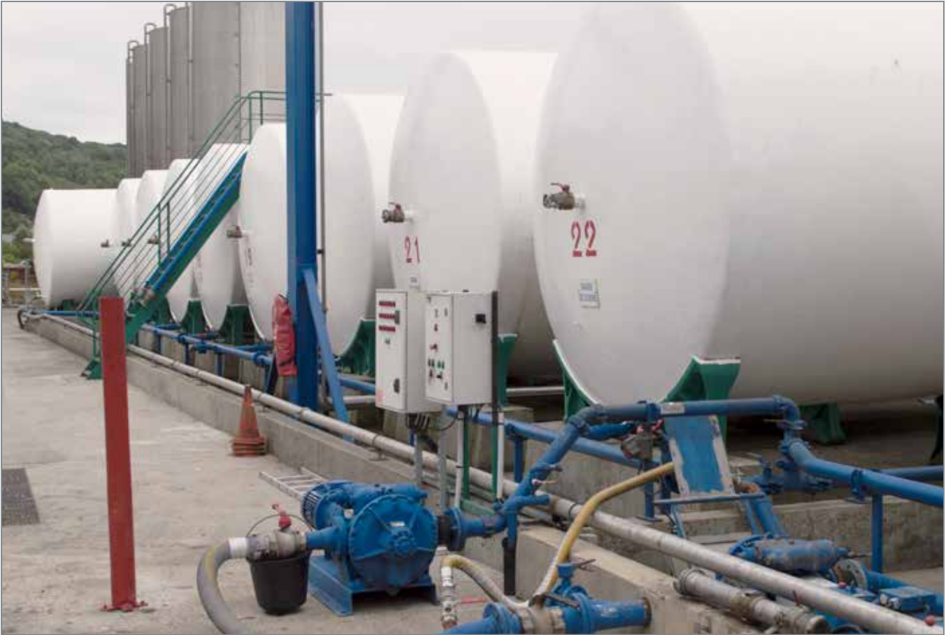
As part of its process, OLVEA Group utilizes large storage tanks to house the oil prior to transferring it to 330-gallon IBCs and 50-gallon drums.
