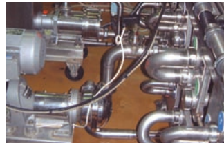
S4C FOR CONDITIONING
