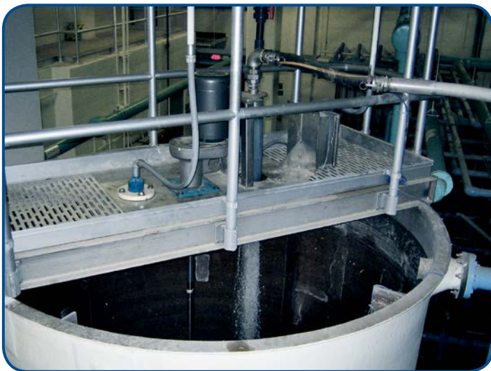
Many operational variables and characteristics must be considered before selecting a mixer. These include mixer type, fluid viscosity, rate of agitation, tank shape and volume, and pumping rate.
